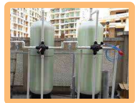
Water Treatment Softener Plant
